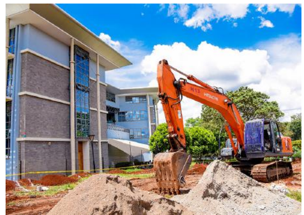
➤ Ground-breaking ceremony for the upcoming APHRC Training Center on November 14. The training facility, scheduled for completion November 2019, will be home to young and upcoming experts seeking to strengthen their research skills.
